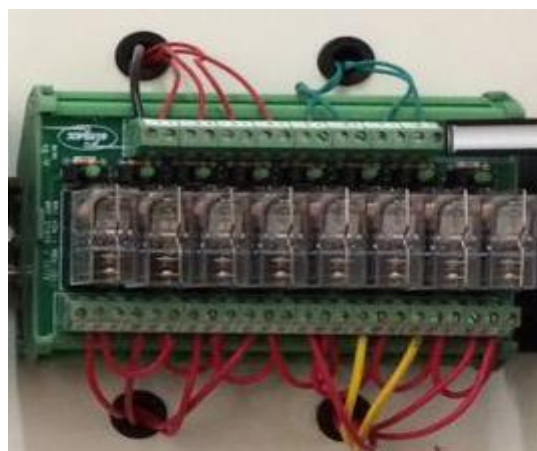
Fig Relay Unit.
